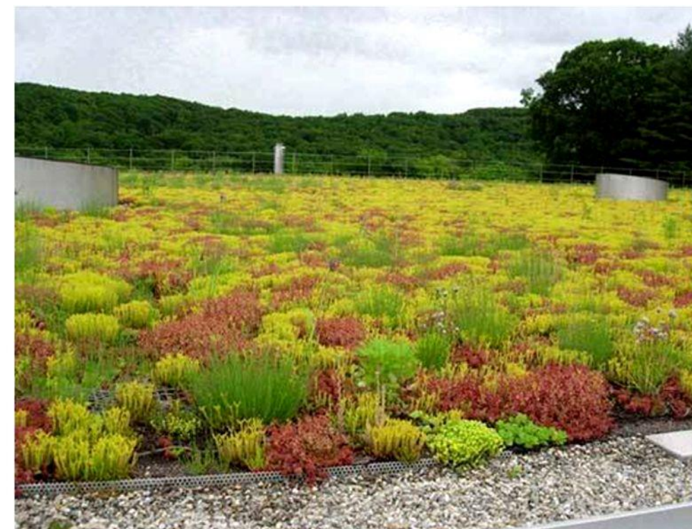
The green roof covering the Whitney Water Treatment Plant in New Haven is the largest in the state at 30,000 sq. ft. © Greenroofs.com
