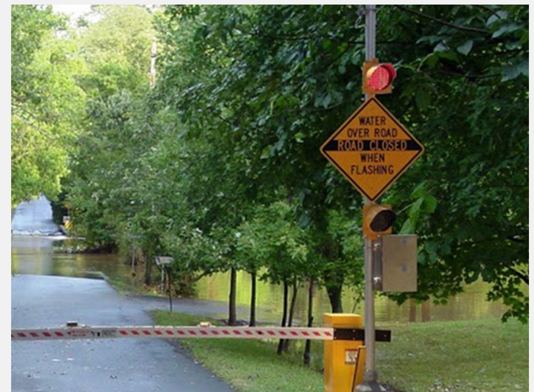
Source: High Sierra Electronics. The top image shows a warning system with no gate, while the bottom image includes a gate.
