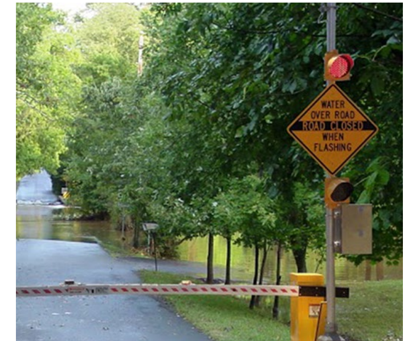
Source: High Sierra Electronics. The image shows a warning system with a roadway gate.
